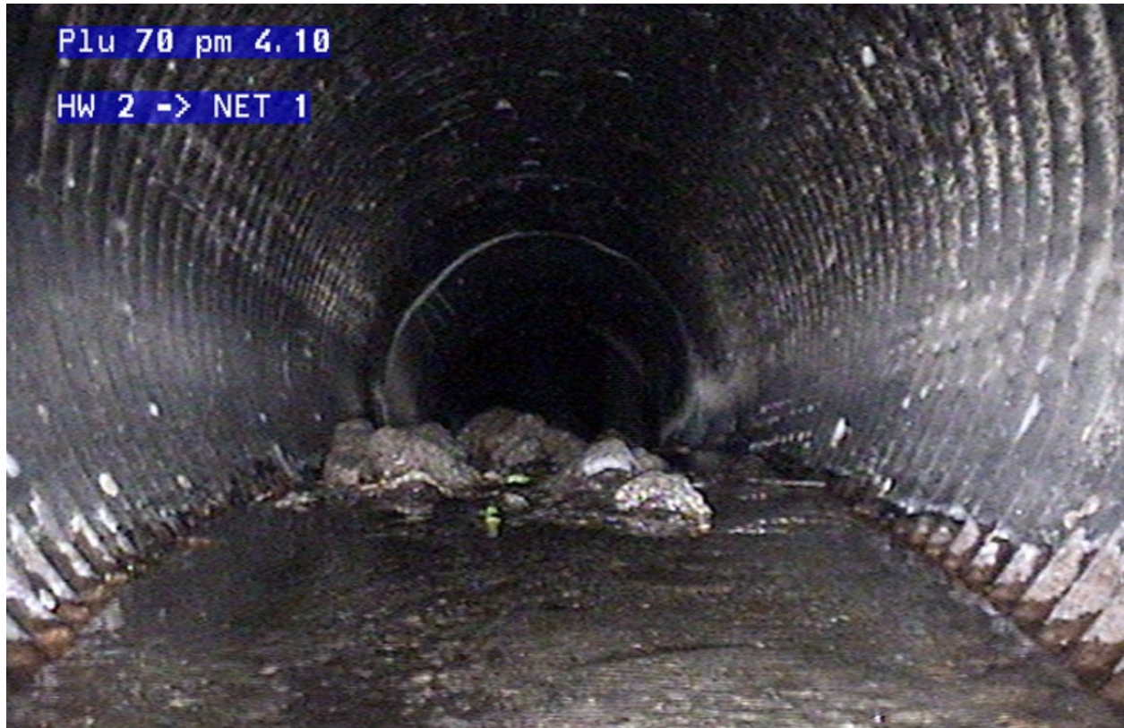
Current conditions of a water passage on State Route 70 in Plumas County
